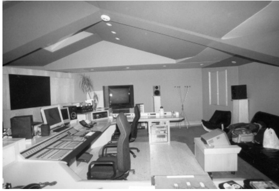
Figure 12.10 The ‘Kyoto’ control room at Eurosonic, Madrid, Spain, designed by Sam Toyashima. The room is used for mixing stems for film soundtracks. The surround loudspeakers are pedestal mounted at the sides and rear of the room. The large, right-front monitor is the black rectangle at the left of the photograph. The console-mounted loudspeakers are for stereo television mixing
